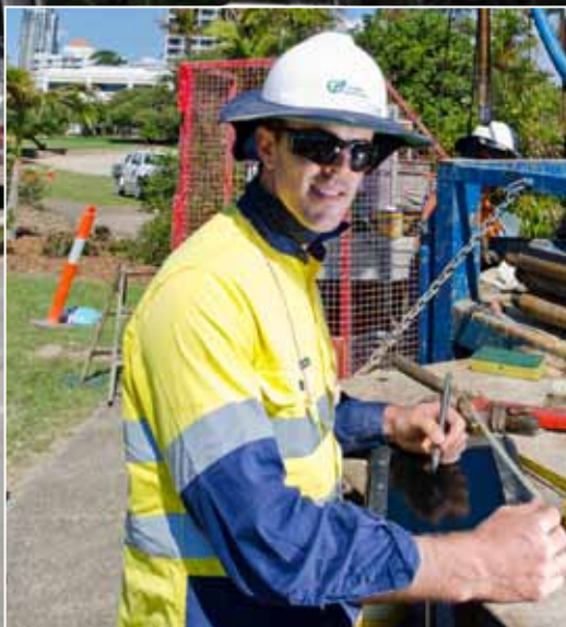
Undertaking geotechnical activities during the project's early works. Images courtesy of the Gold Coast Rapid Transit project.
