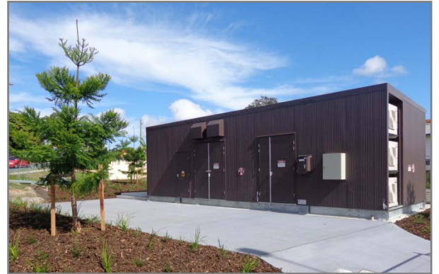
Traction Power Substation
