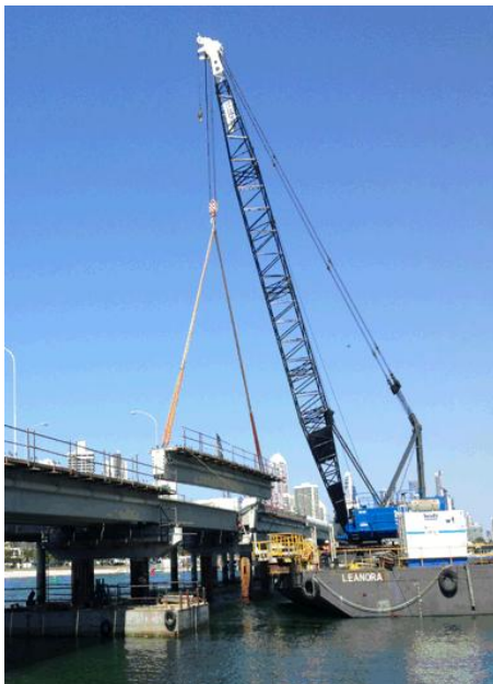
The final girder lift for the light rail bridge across the Nerang River
