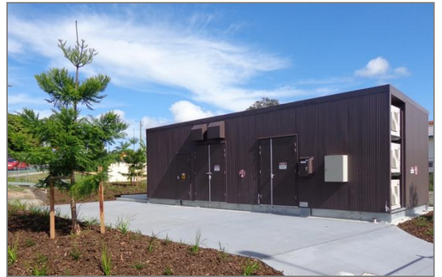
Traction Power Substation
