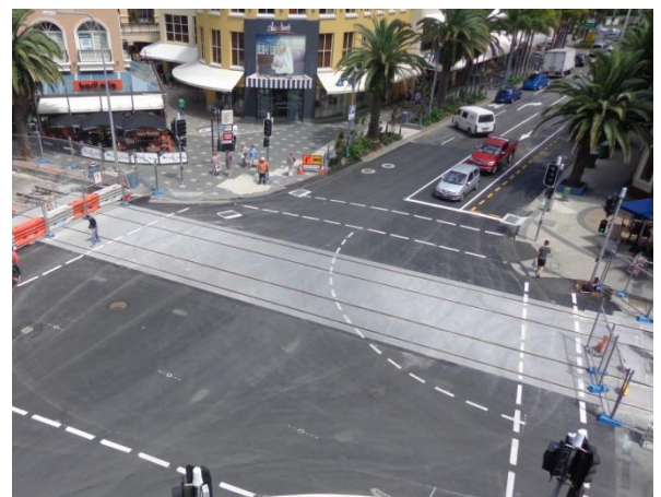
First track installed in Surfers Paradise at Surfers Paradise Boulevard and Elkhorn Avenue intersection
