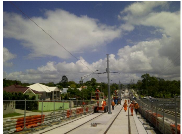
First look at the overhead lines at Queen Street
